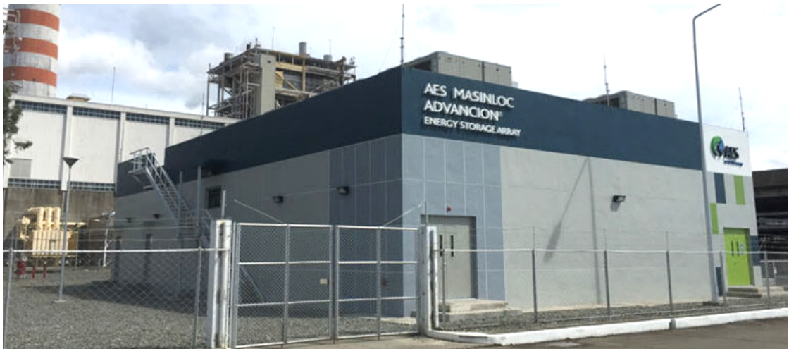
Photo: AES Energy Storage Array in Masinloc, Zambales. Image from Technocrete Trading.
